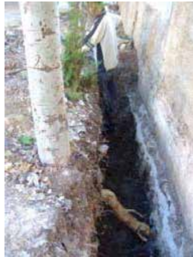
Image (4) Deep-Rooted Poplar Tree Penetrating the Foundation Soil of a Building (7)
